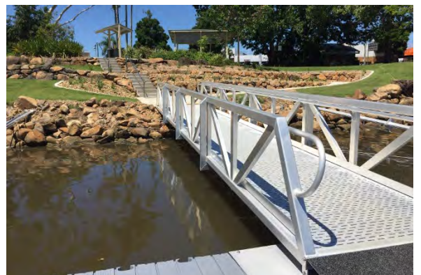
Figure 3 Pontoon and gangway installation with disability access ramp at Budd Park, Murwillumbah.
