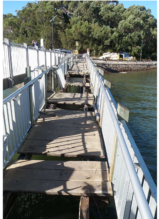
Figure 1 Storm damage on the access way to the Bundeena public wharf. Photo courtesy of Sutherland Shire Council.
