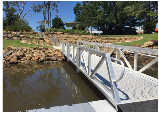
Figure 3 Pontoon and gangway installation, as well as disability access ramp to the gangway, at Budd Park, Murwillumbah, along the Tweed
